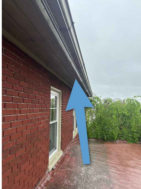
Peeling paint on wood soffits and fascia
