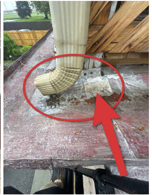
Flashing above may be allowing water to leak into soffit
