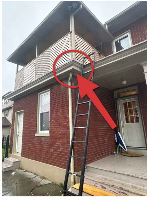
Wood soffit rotted
