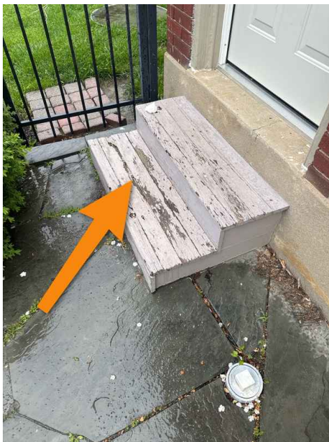
Step boards beginning to rot
