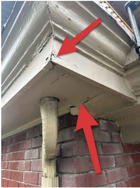
Close up of wood rot
