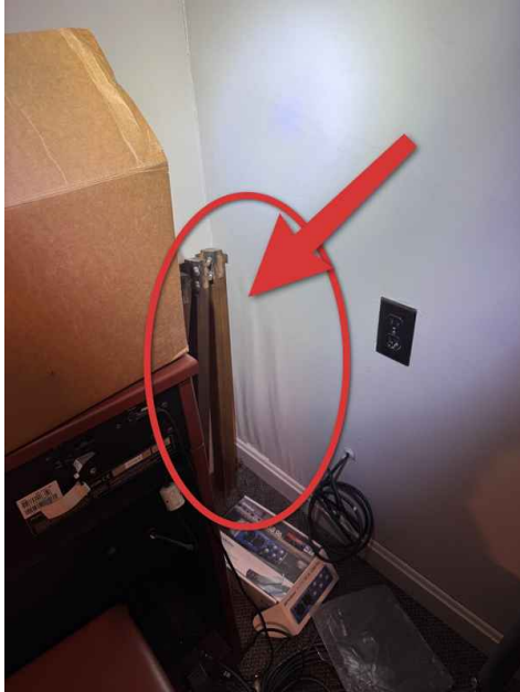
Drywall is wet
