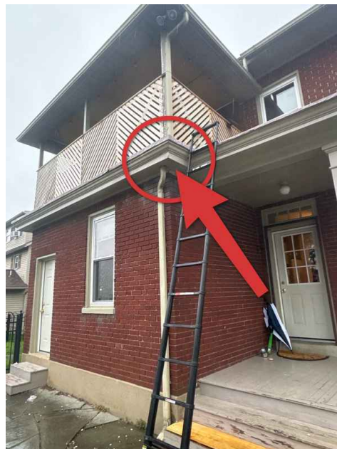
Wood soffit rotted
