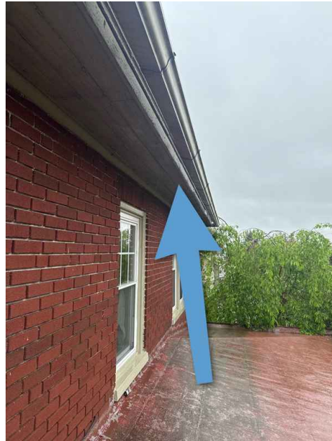
Peeling paint on wood soffits and fascia
