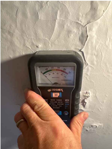
Currently dry on moisture meter
