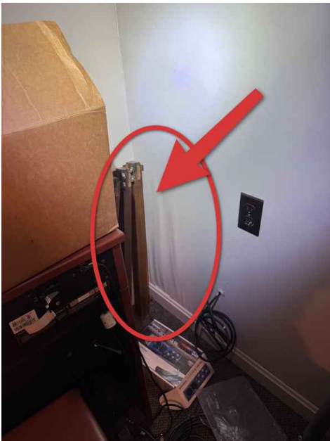
Drywall is wet
