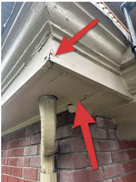
Close up of wood rot
