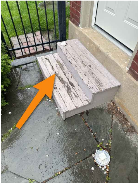
Step boards beginning to rot
