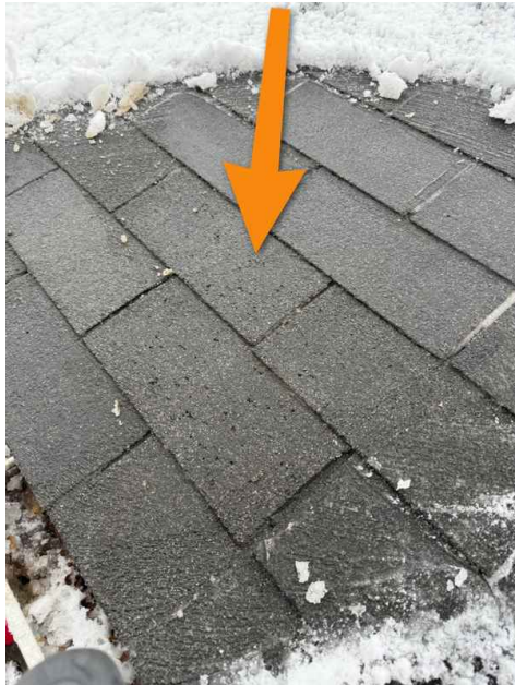
Shingles appear worn
