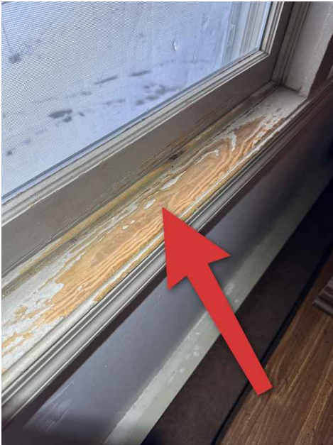
Significantly worn window sill
