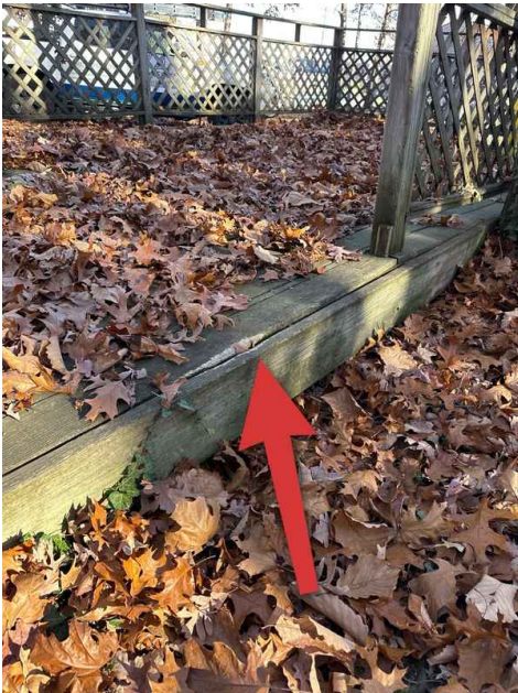
Grade level deck potential invisible defects
