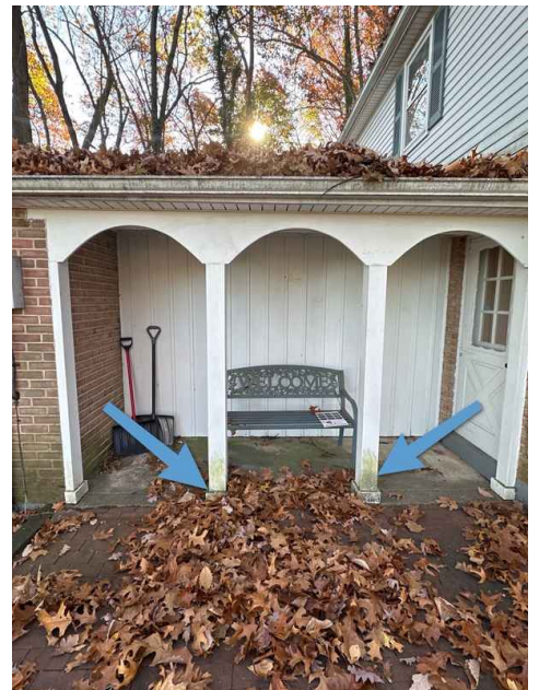
Loose at base
