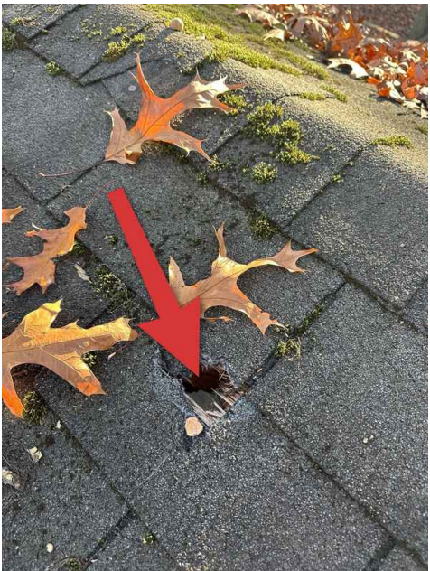
Hole in roof Garage
