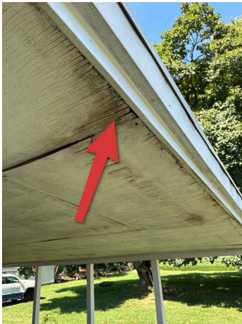
Rotten porch ceiling plywood
