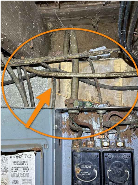
Representative of wiring Throughout
