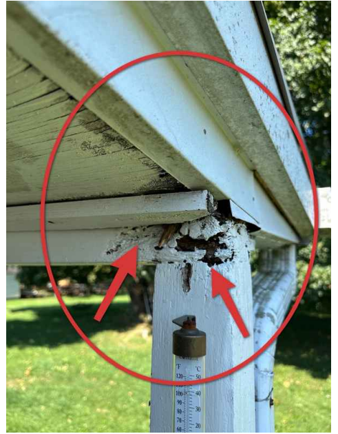
Rotten post and carrier beam
