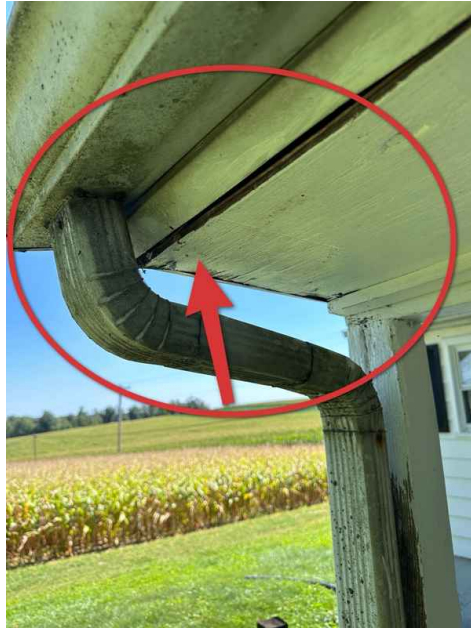
Softening soffit member
