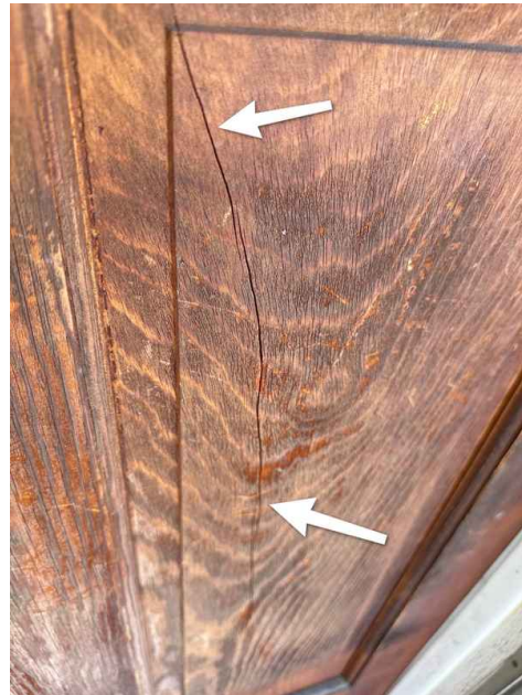
Close up of split panel
