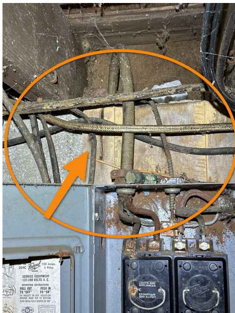
Representative of wiring Throughout
