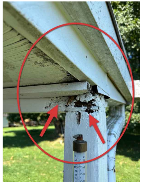
Rotten post and carrier beam
