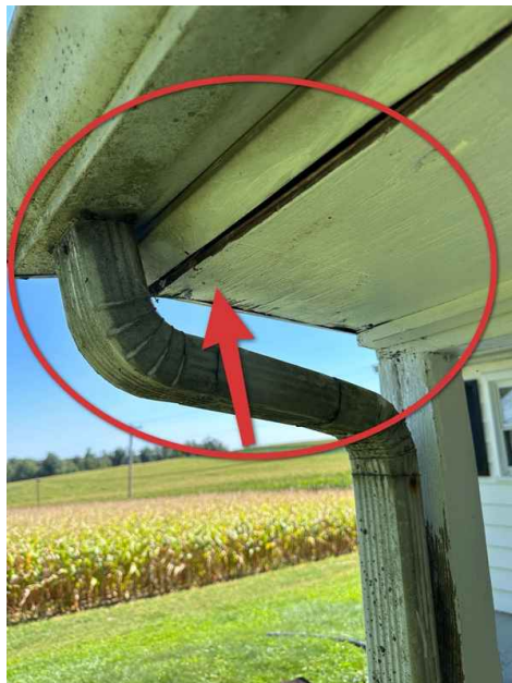
Softening soffit member
