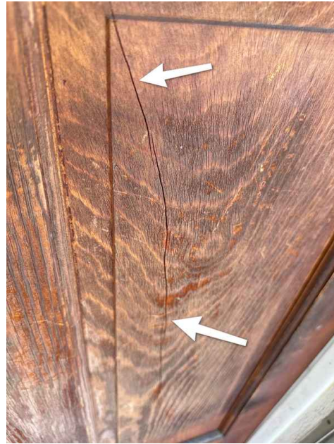
Close up of split panel
