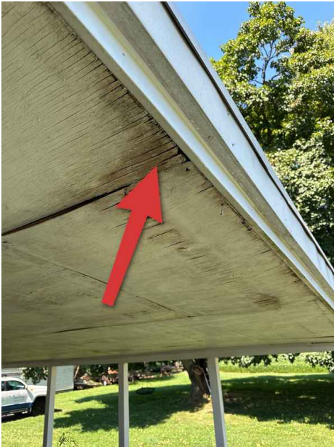
Rotten porch ceiling plywood
